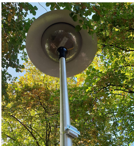
FIGURE 5 | Beacon mounted in lamppost.
