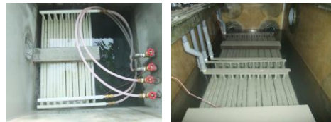
Figure 3 Heat exchangers soaking in tanks
