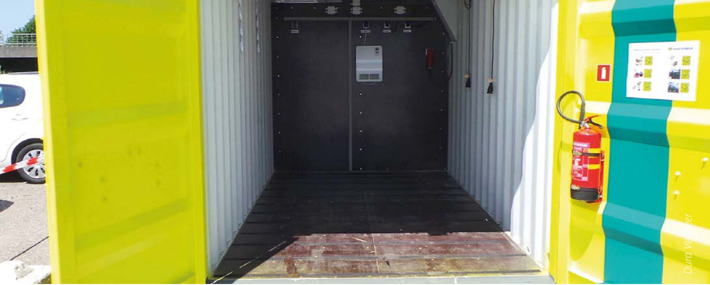
Mobile charging container for electrical equipment from Dura Vermeer
